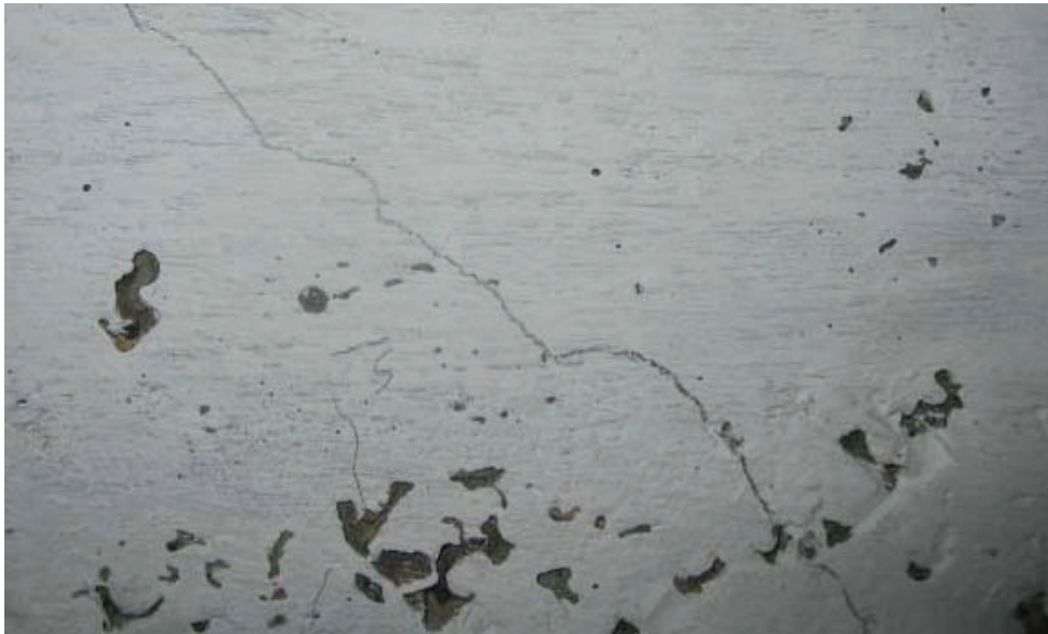
Figure 8. Flexural cracks induced under UDL
